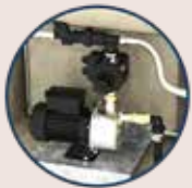
Pump pre-installed with rain/mains changeover
